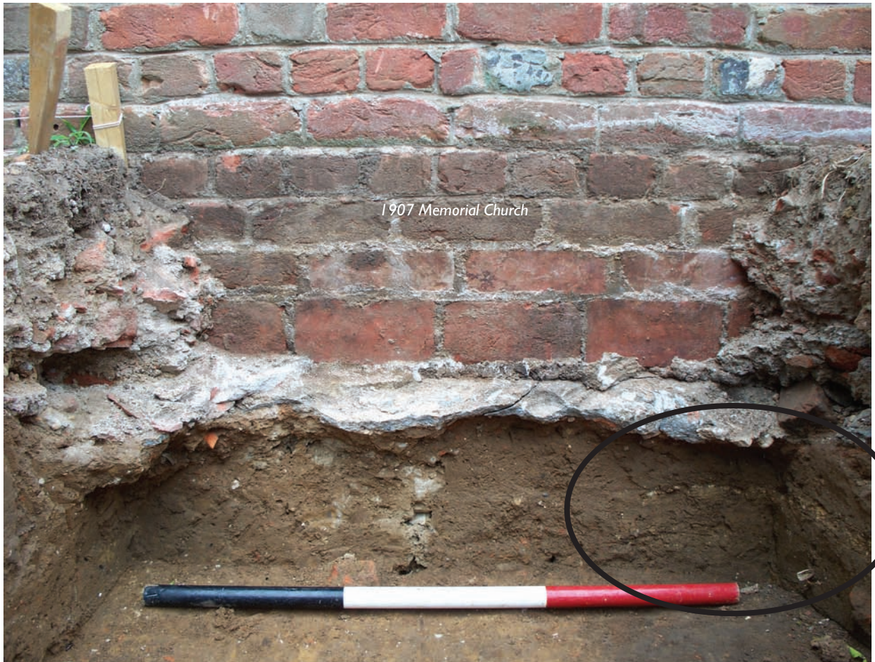
Figure 134. View of Memorial Church foundations and sand mortar band, as indicated by black oval (facing west)
